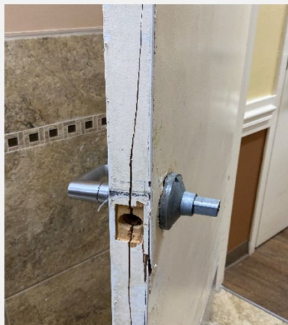
10. Broken Bathroom Door
