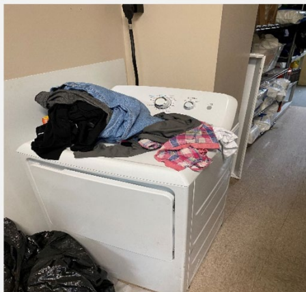
11. Dryer With No Vent
