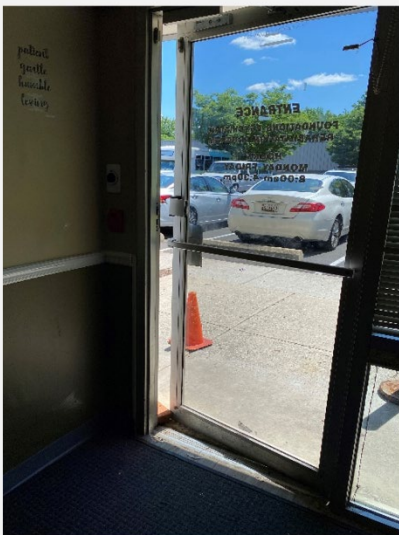
5. Exit Door Propped Open
