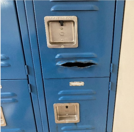
13. Hole in Locker
