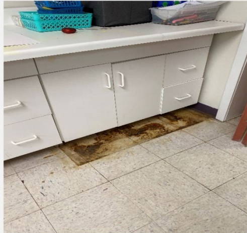
14. Missing Floor Tile
