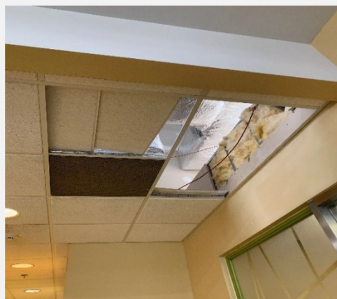
12. Missing Ceiling Tile
