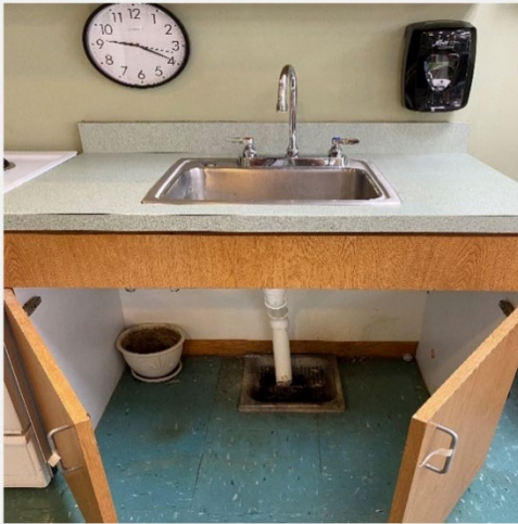
17. Dirty Drain Under Sink
